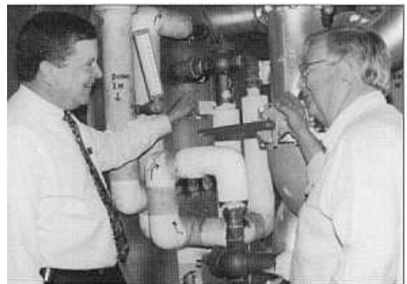
John Sams (left) of Heat Transfer Sales discusses the Heat-Timer Tempering Valve installation with Bud Bodenheimer of Bodenheimer Plumbing Services, Inc.
