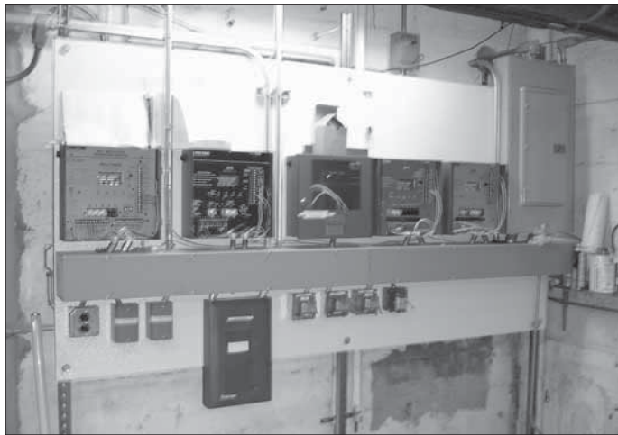
Each Heat-Timer control provides unique adjustment capability to maximize the efficiency of each individual system. Remote communications allows for local and/or remote adjustments.
